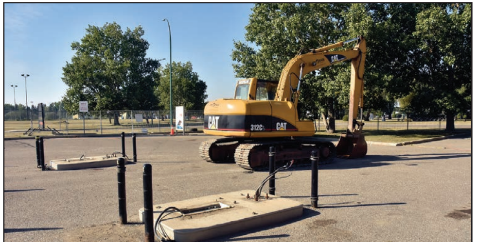
There's a new look to the ESSO gas bar offered at CANEX following construction that started last summer (above), and was finished last month when the lights were installed (top). Photos Jules Xavier
