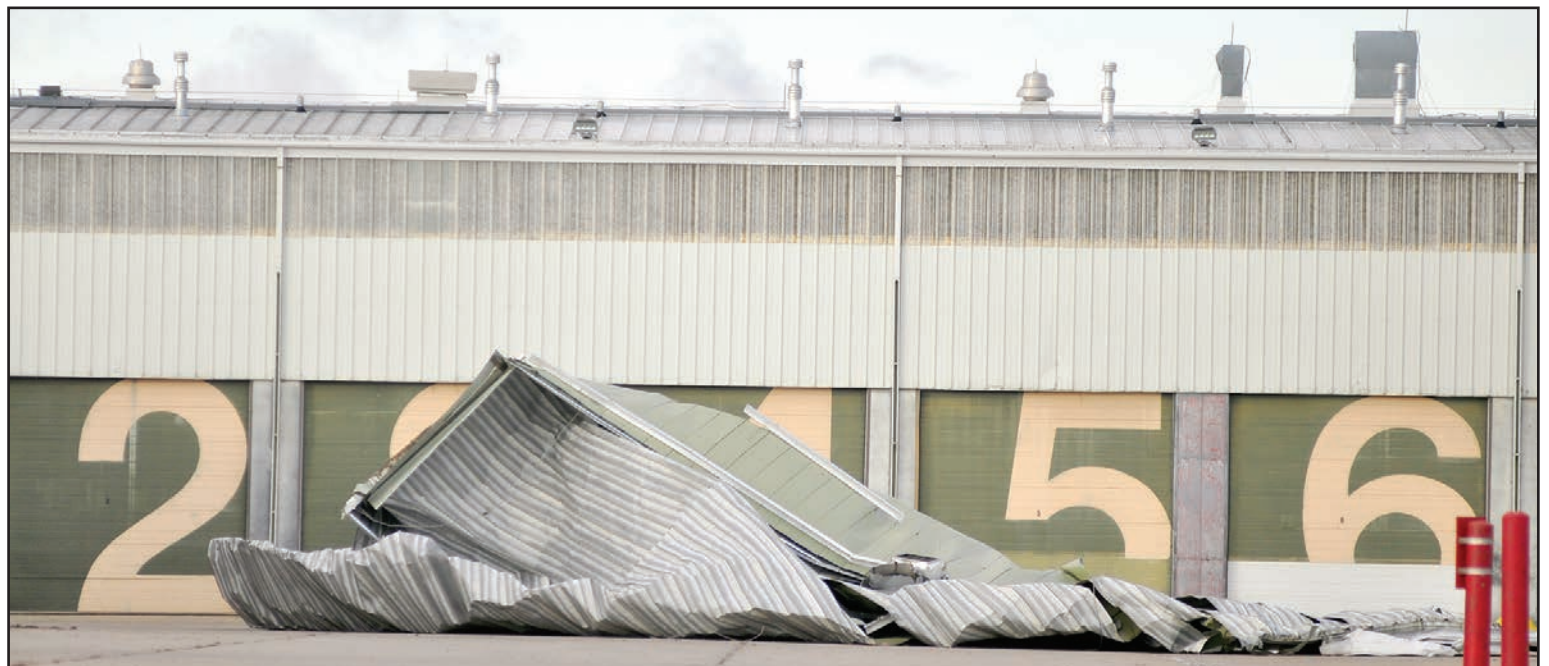
A section of the roof peeled off by heavy prairie winds sits on the ground in front of an adjacent Base Transport building.
