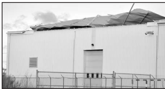
A section of Base Transport's roof on west side of building is peeled back.
