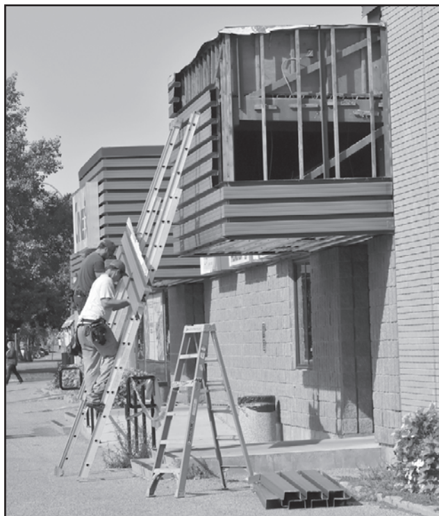
Workers remove the siding from one of two canopies which are part of the renovations being done to CANEX. Jules Xavier/Shilo Stag
