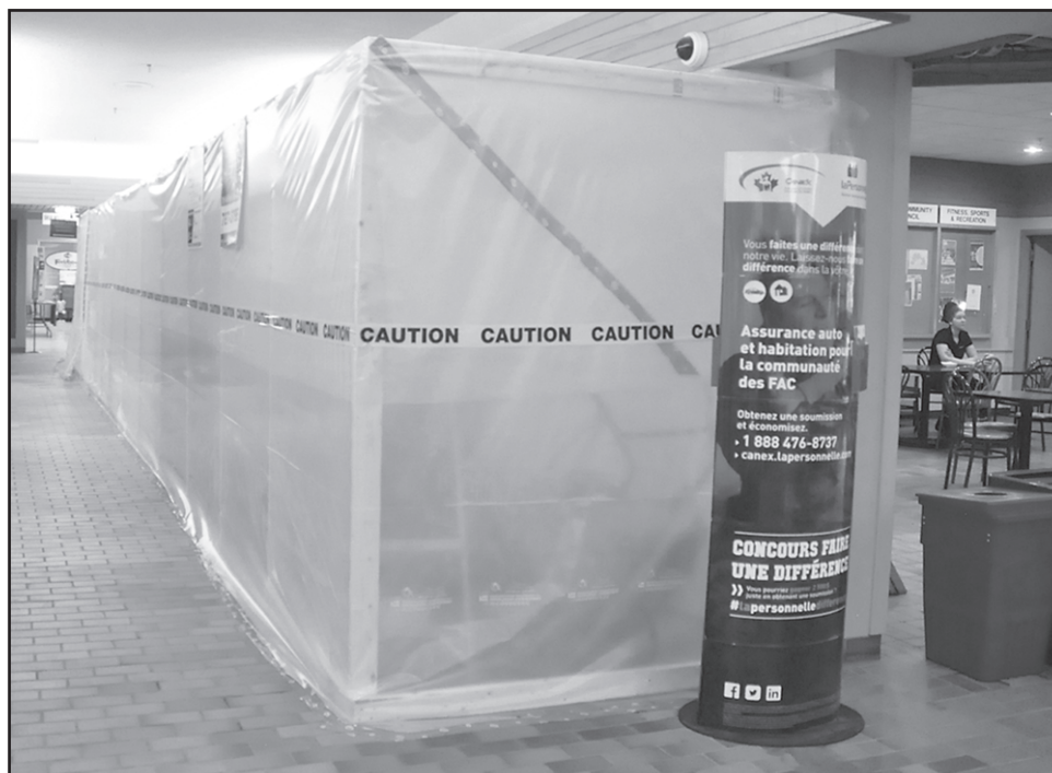
A section of the CANEX interior is blocked off to allow work on a section of the flooring. The entrance to the Stag's office is accessible through the plastic covering while work is done after the building has closed.
