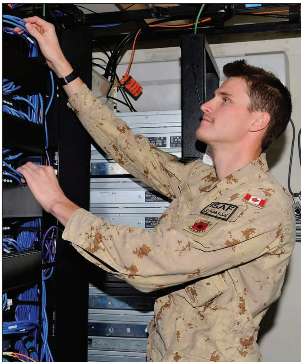
MCpl Matthew Hall, a signals operator with the National Command and Support Element, inspects a cable router at Camp Phoenix, Kabul in early November.
