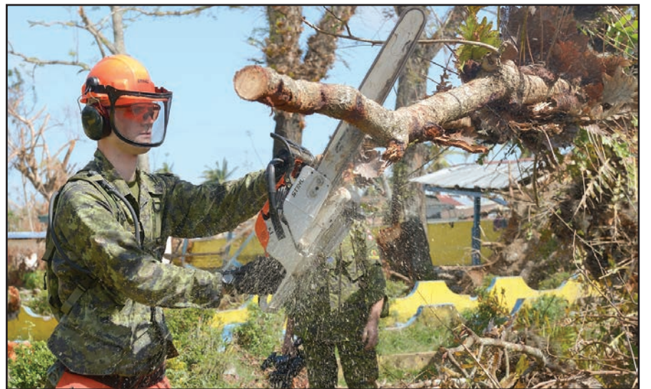
Private Justin Williston, combat engineer with the Disaster Assistance Response Team (DART), cuts a tree blocking the way to Dona Victoria Cortes Dais Memorial School in Pontevedra, Philippines on Nov. 19, 2013.
