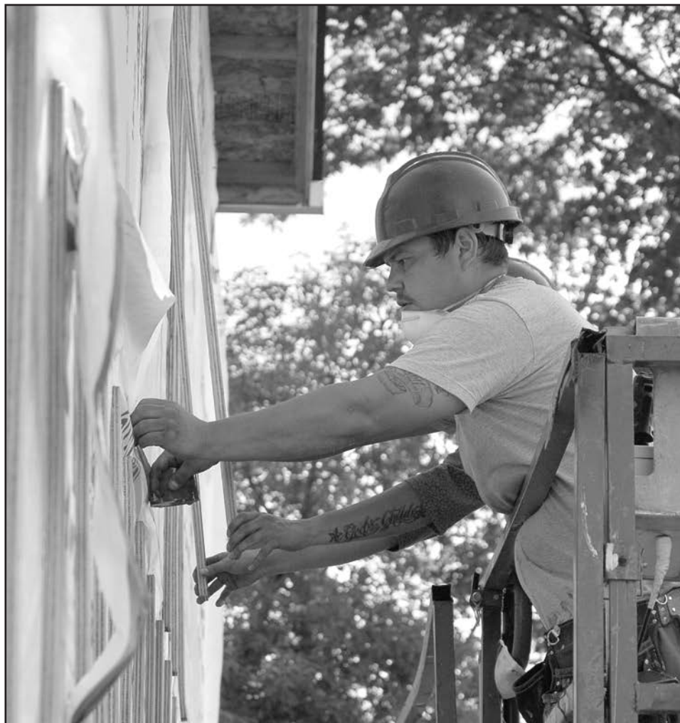
Work on replacing old RHU siding is underway this summer as part of improvements to CFB Shilo's RHUs. Here, two workers prepare an exterior wall on a duplex for the new siding. Photo by Cpl Janie Jacobsen
