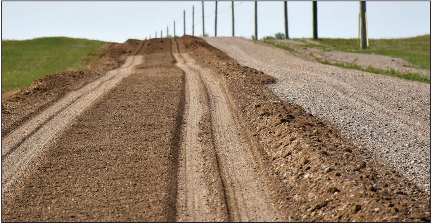
A segment of road out to the training ranges which has been dug up. It's waiting for a treatment to help prevent dust from rising when vehicles pass over during training exercises.
