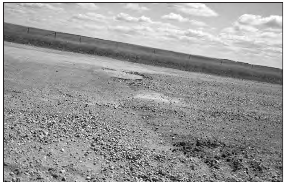
Point of contention: the point where the smooth pavement abruptly turns to dilapidated gravel road.
