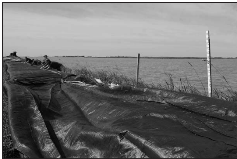
Aquadams placed against a wall of water to protect homes and infrastructure. This task, heavily based on A and B batteries is responsible for the preservation of several homes and roads.
