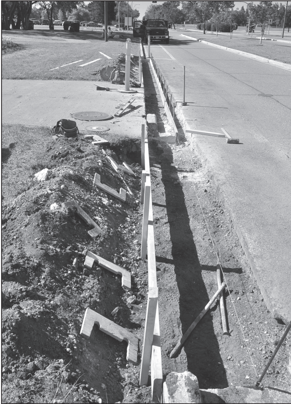
Before paving starts, road crews are busy repairing curbs on Royal Avenue. Photo Jules Xavier
