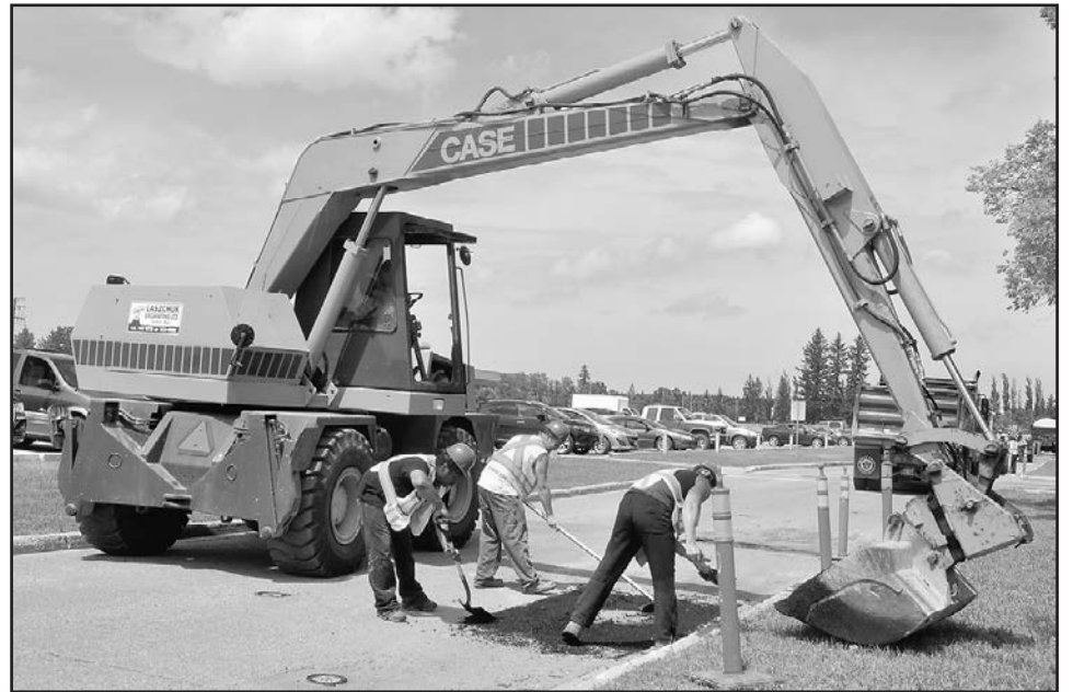
Motorists are reminded to slow down around the asphalt crews currently working on Base roads, like this one in front of headquarters.
