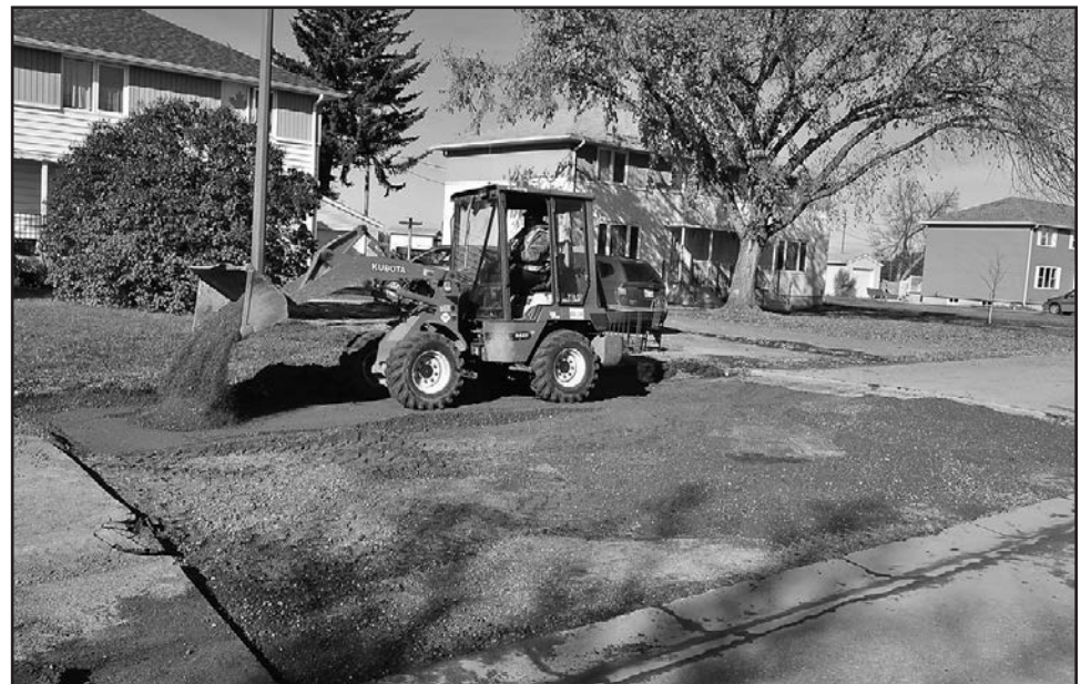
Work repairing Kingston Avenue is underway, with asphalt going down once the ground is levelled. Photo by Jules Xavier
