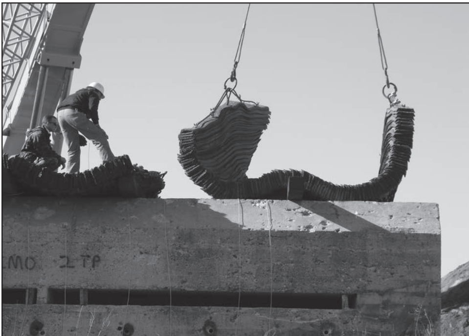
Above, Members of ICER set explosive charges to prepare the bunker for demolition.
